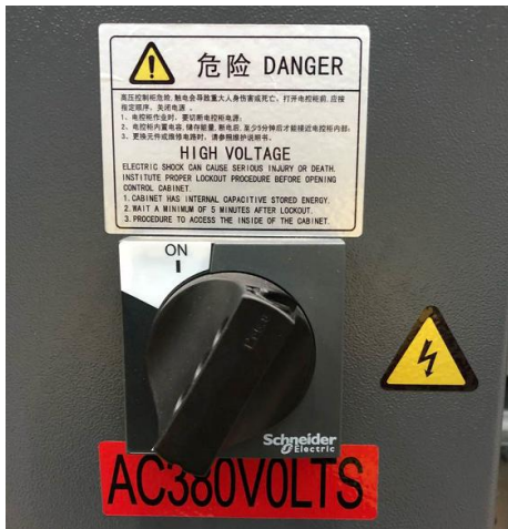
Figure63:Electrical Cabinet ON/OFF switch 电柜 ON/OFF 开关
