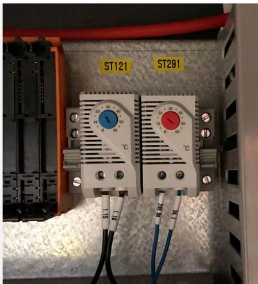
Figure 70: Checking operation of ventilation 检查通风操作
