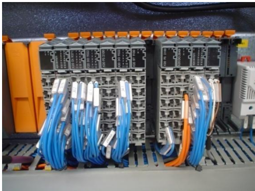
Figure 34: SINCONV connection SINCONV 的连接
