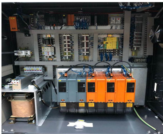
Figure 68: Cabinet interior 电柜内部
