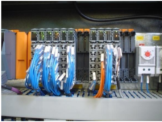
Figure 30: SINCONV connection SINCONV 的连接
