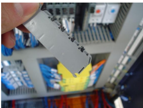
Figure 32: SINCONV connection SINCONV 的连接
