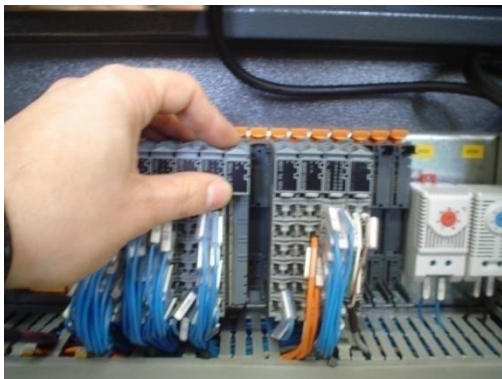
Figure31: SINCONV connection SINCONV 的连接
