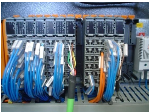
Figure 35: SINCONV connection SINCONV 的连接
